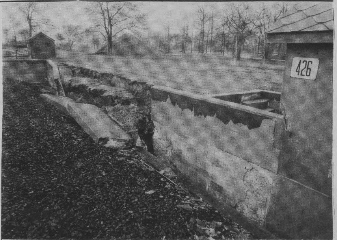
Crumbling walls on one of the College's two trickling-filter tanks emphasize the fact that the sewage treatment plant, which has been in service since World War II, is ready for either retirement or major overhaul (photo by Russ Kowal).
