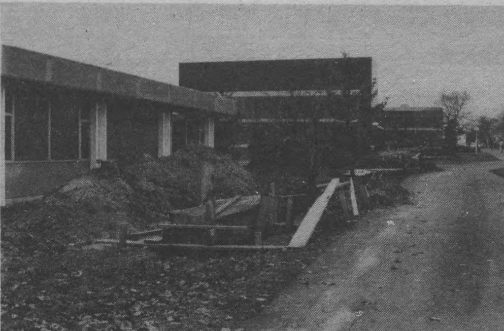
Problem pipes—Heat pipes recently repaired in front of Main Hall could pose a serious problem in the future. The 15 year old pipes are deteriorating and could spring leaks at any time. Workers await the decision for change in the system before covering the pipes.
