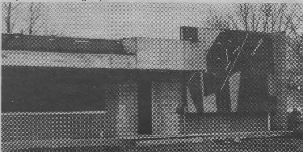
Construction is proceeding on the future site of the latest Quick Chek Food Store which is scheduled to open in April, across the street from the College.
